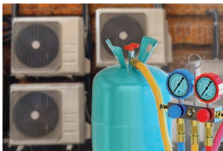
Verification of gas pressure
