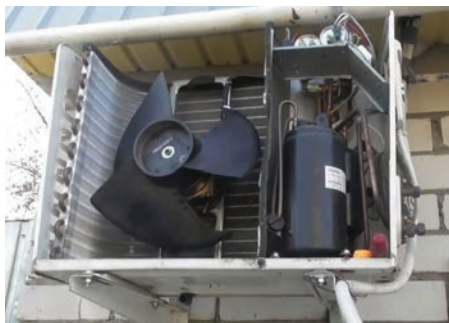
Exchanger and compressor
